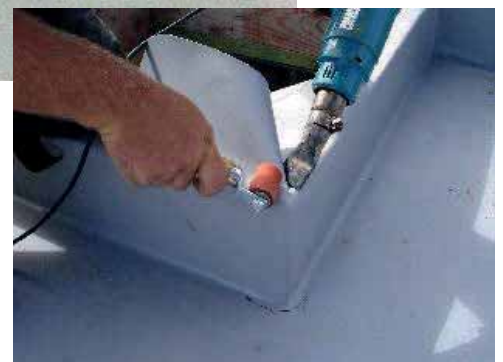
Automatic and hand welder
