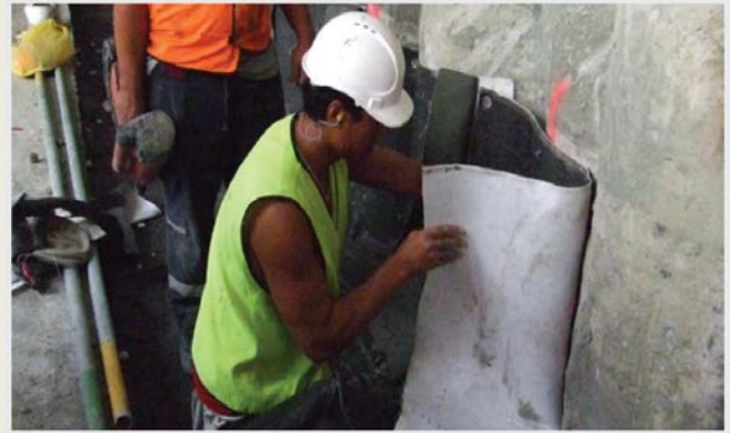
Above: rawMAT being installed to the piles of the Deloitte Centre (BNZ Building) on Queen Street, Auckland
