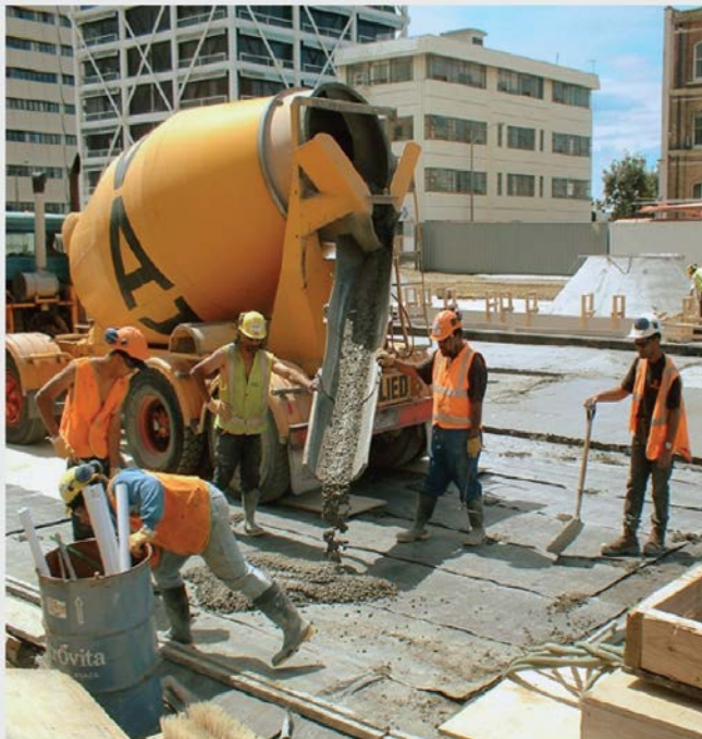
Above: rawMAT installed onto the roof of the Britomart transport centre, Auckland
